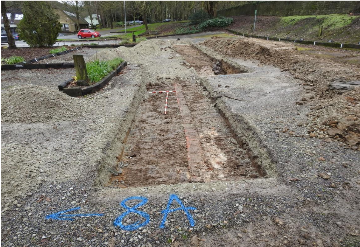
Plate 15: Showing Trench 8A and retention wall in foreground. Looking east with one- and two-metre scales.
