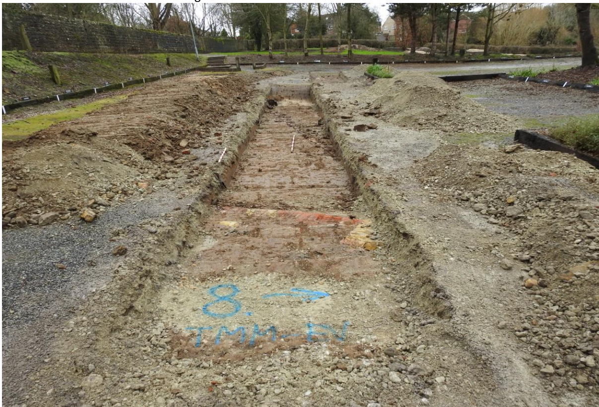
Plate 14: Trench 8 looking west. Slightly curving retention wall visible in foreground. Ceramic pipe visible in background. Looking west with two-metre scales.
